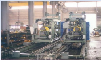
<Cr COATING 설비>
